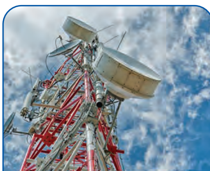
Telecom -Data Infrastructure
